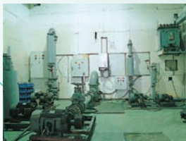
Testing area for Roots Blower
